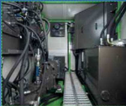
Service-friendly designed engine room Servicefreundlich gestalteter Maschinenraum
