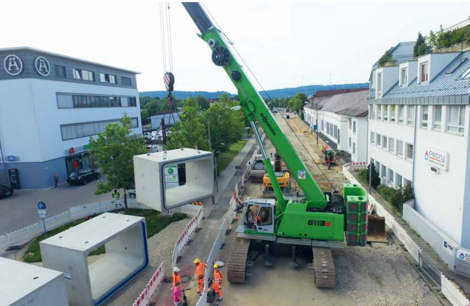
26 6113 R - moving and positioning large and heavy components in civil engineering; Germany
