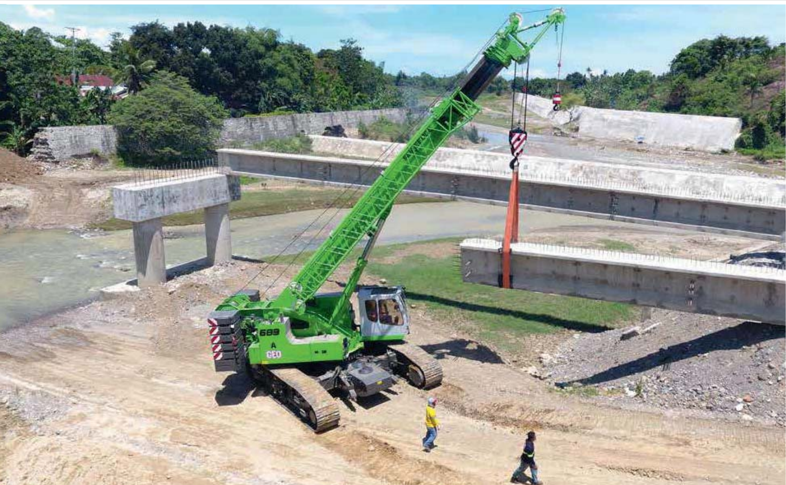
683 R – infrastructure pre-fab concrete parts, pick & carry operation; Philippines 683 R - Infrastruktur Betonfertigteile; pick & carry; Philippinen
