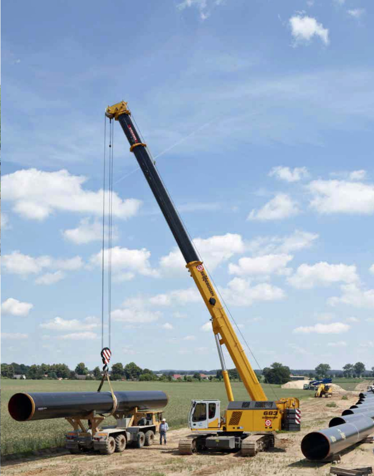
683 R - installation of large pipe thanks to Pick & Carry 683 R - Pipelinebau dank Pick & Carry Einsatz
